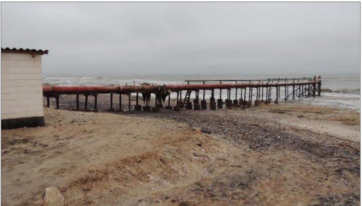
Figure 19: Survey Site 4: View west from the proposed intake point depicting the existing salt works intake structure.
